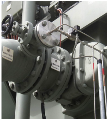
Connection to collect the Oil
