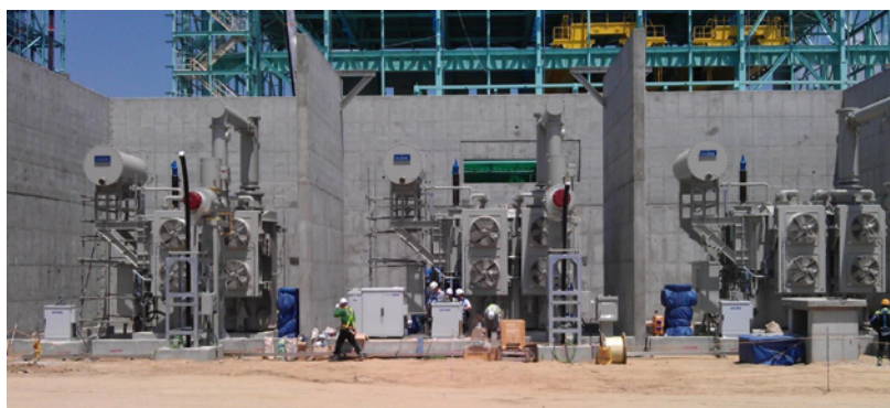
OnlineDGA for 3 Transformers
